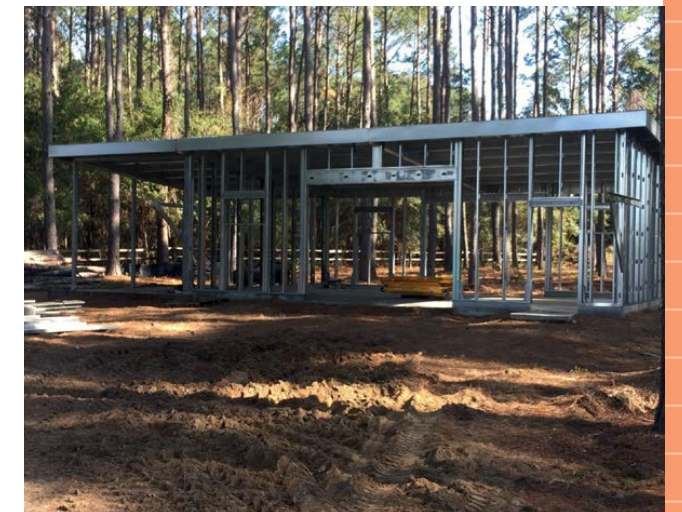
Above: The frame was installed atop the pilings prior to the insulation and metal panels. (Photo courtesy of EcoSteel.)
